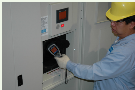
Technician scans the interior of a Powersmiths Energy Station™ PDU through the Rotatable IR Port with recessed mount as part of a preventative maintenance program.
